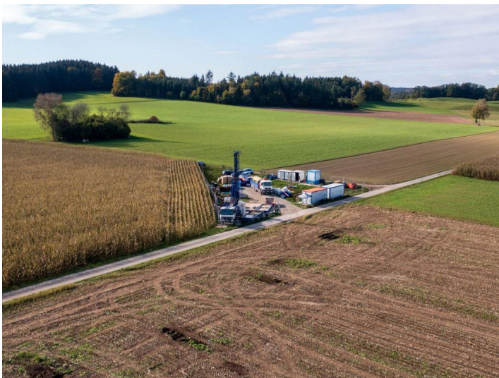
Drilling tillites deposited in overdeepened valley at the Tannwald site nearby Winterstettenstadt.
