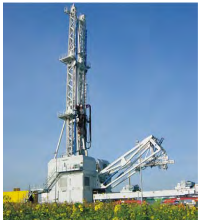
Figure 1. InnovaRig with hydraulic pipe handling unit on lower right side. Photo by Herrenknecht Vertical.
