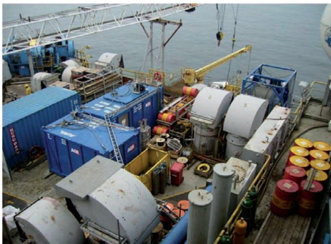
Figure 5. The AGR riserless mud recovery system deployed on an oil and gas exploration vessel.
