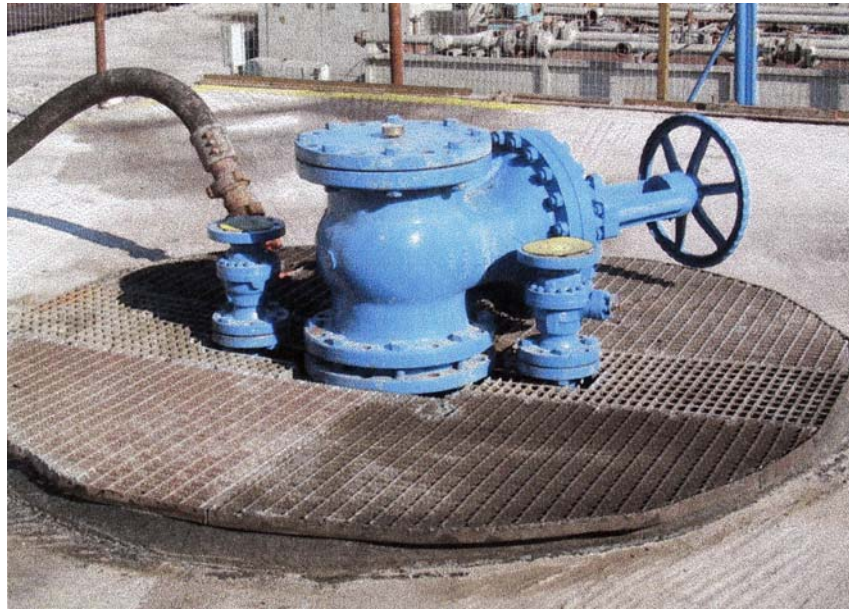
Fig. 5. Wellhead of the AIG-10
