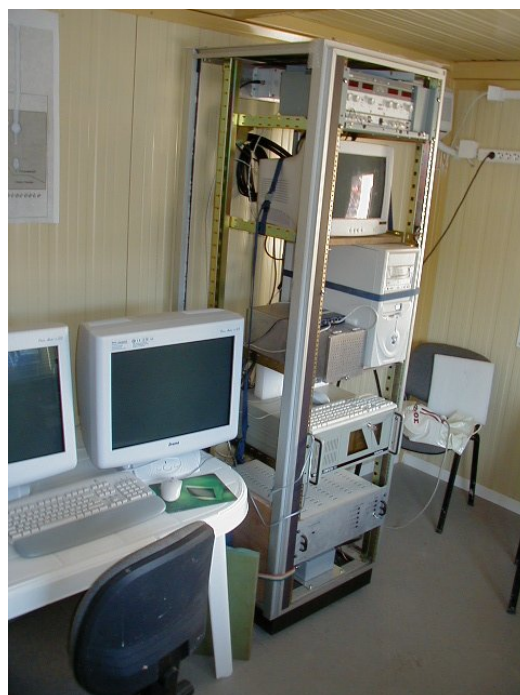
Figure 6. The data acquisition system as installed in the shelter in Aigion. Presently the structure is tightened to the shelter frame in order to prevent it from falling in case of strong earthquake.
